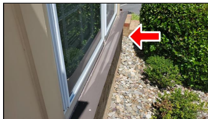
8.0 Item 1(Picture) Example/ Sample- Front of home- Sill slope improper
