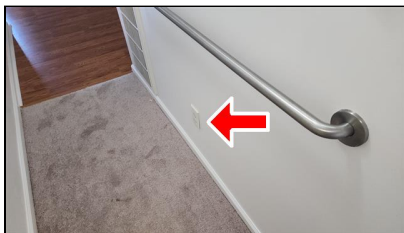
3.5 Item 1(Picture) Example/ Sample- Hallway- Loose outlet
