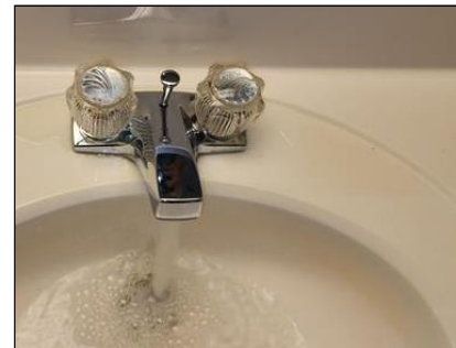
2.4 Item 4(Picture) Example/ Sample- Primary Bathroom Sink- faucet leaks while in use
