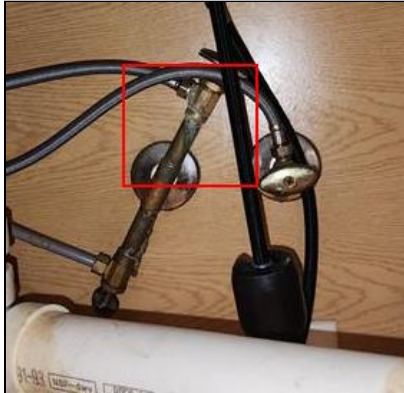
2.4 Item 1(Picture) Example/ Sample- Kitchen Sink
