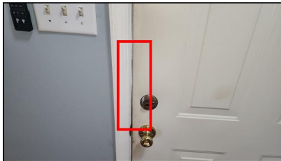
1.2 Item 1(Picture) Example/ Sample- Front Door- Exterior door(s) – weather-stripping- missing
