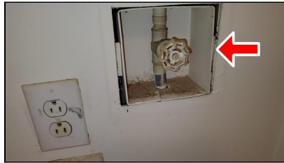
2.2 Item 1(Picture) . Interior cut off located in the washer dryer area.
