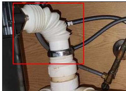
2.4 Item 3(Picture) Example/ Sample- Kitchen- corrugated drain line
