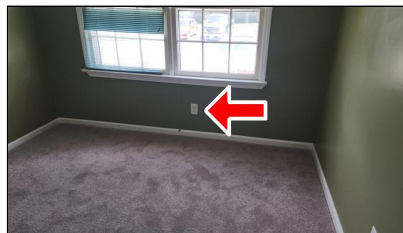
3.5 Item 2(Picture) Example/ Sample- Front Right Bedroom- Loose outlet
