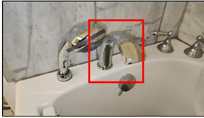
2.4 Item 5(Picture) Example/ Sample- Primary Bathroom Tub- faucet loose
