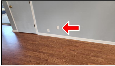
3.5 Item 4(Picture) Example/ Sample- Living Room- Ground connection missing
