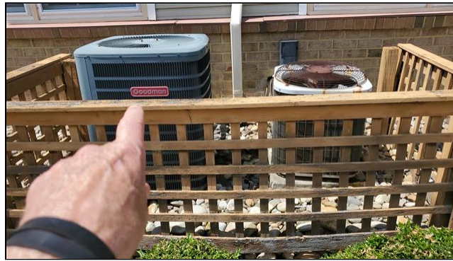
Outside HVAC condenser location
