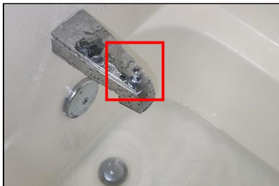
2.4 Item 2(Picture) Example/ Sample- Hall Bathroom Shower- diverter leaks while engaged, has to be held in position for shower mode
