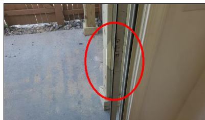
1.2 Item 5(Picture) Example/ Sample-screen door to patio missing handle and the screen is damaged
