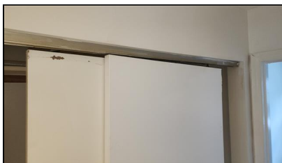
1.2 Item 4(Picture) Example/ Sample- Primary Bathroom Closet- Closet door does not open properly, rubs floor, and/or not in track
