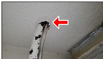
1.0 Item 1(Picture) Example/ Sample- closet area where HVAC air handler located
