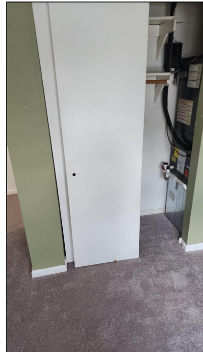
1.2 Item 3(Picture) Example/ Sample- Front Right Bedroom Closet- Closet door does not open properly, rubs floor, and/or not in track
