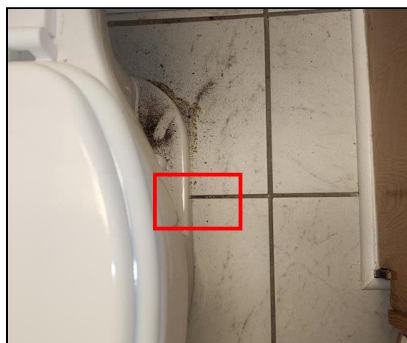
2.3 Item 1(Picture) Example/ Sample- Primary Bathroom- toilet leaks at floor
