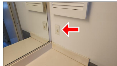
3.5 Item 3(Picture) Example/ Sample- Primary Bathroom- Loose outlet
